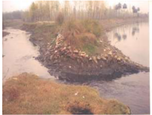
Washed away portion of ditch drain polluting water of Western Jamuna Canal
